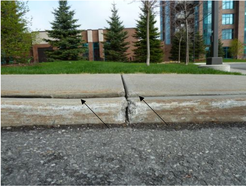
3. Elevation difference between concrete sidewalk and curb near OCSCC 667. This is a tripping hazard.
