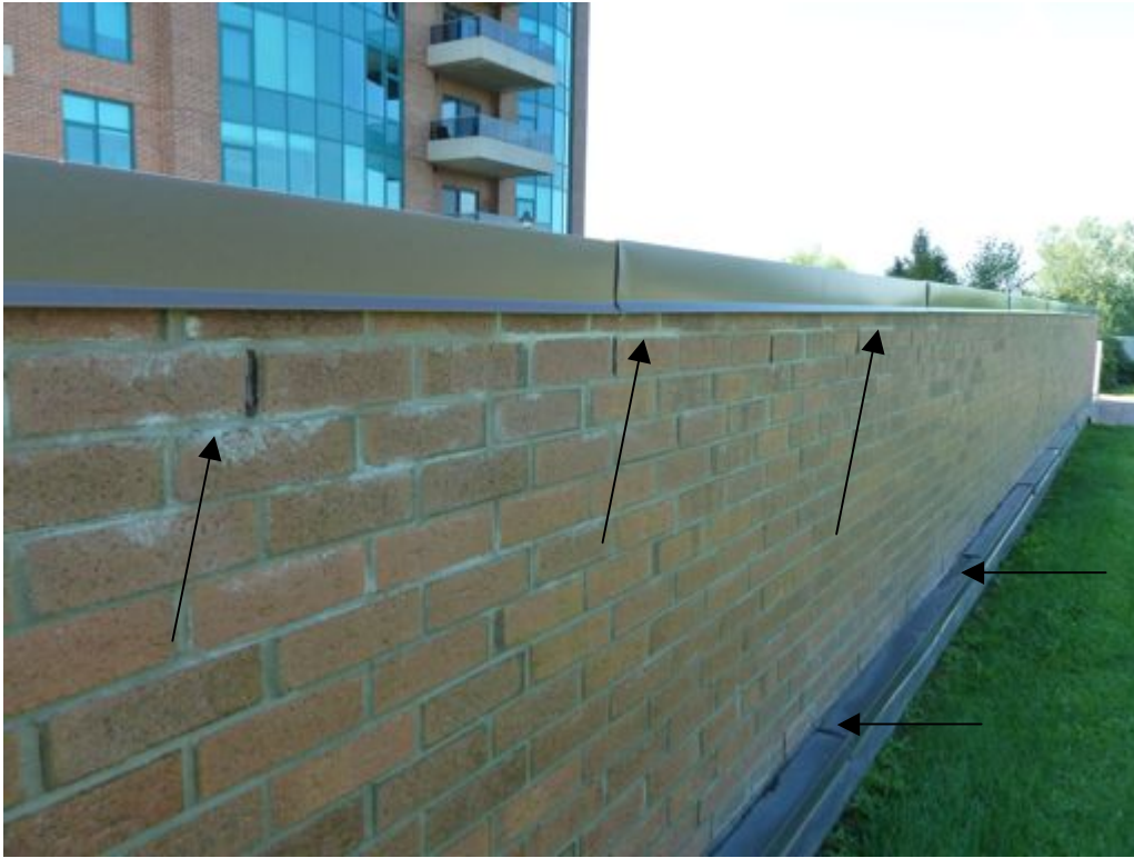
5. Efflorescence on the masonry veneer on the north wall of the Shared pool building. Also note the negatively sloped flashing at the base of the wall.
