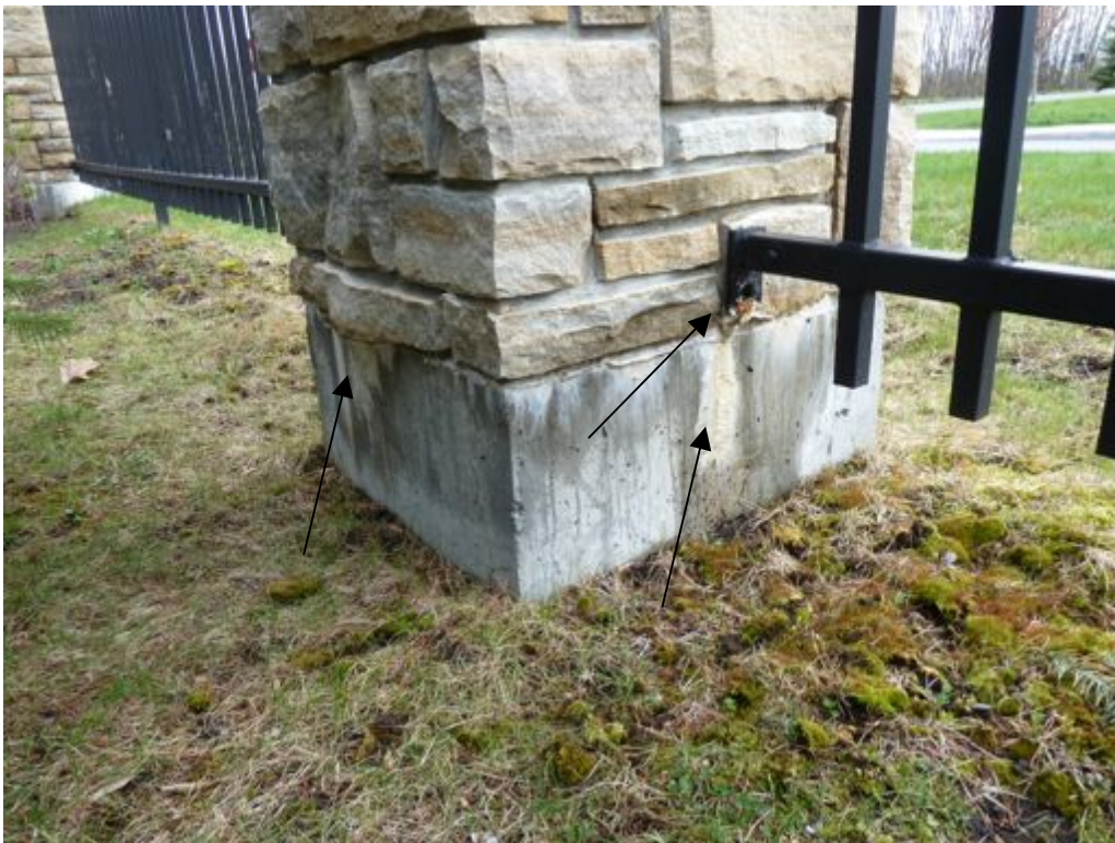
4. Typical masonry fence column. Note the efflorescence at the bottom of the masonry. Also note the steel fencing is corroding at various locations.
