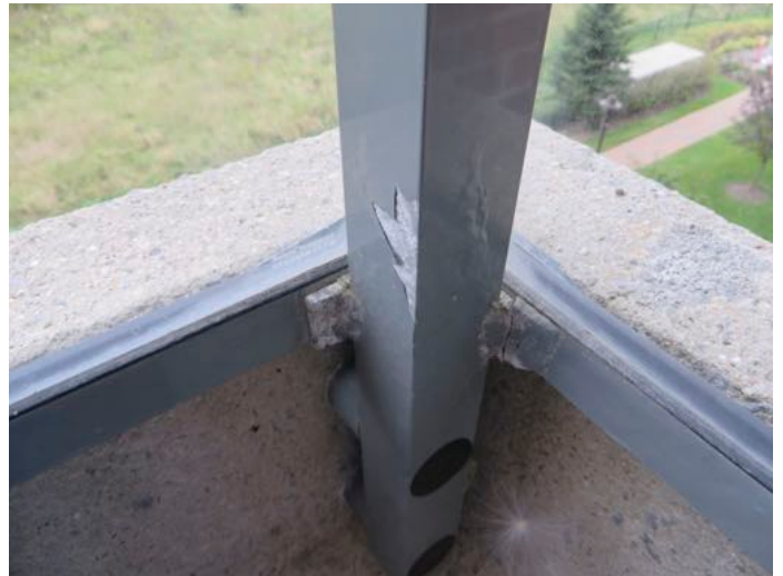
Photo 4 Balcony guardrail example showing peeling paint, corrosion and a cracked member.
