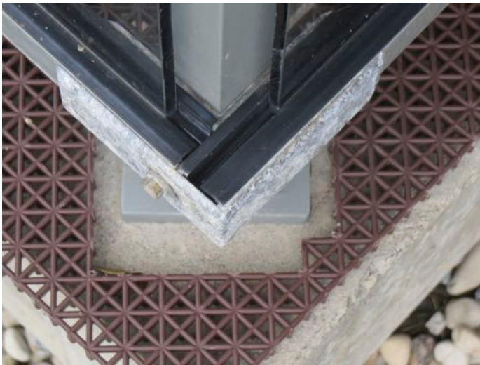
Photo 3 Example of balcony guardrail missing paint due to corrosion.
