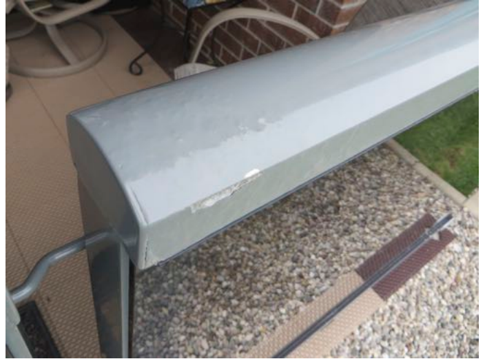
Photo 2 Example of bubbling paint on a pre-finished aluminum guardrail.
