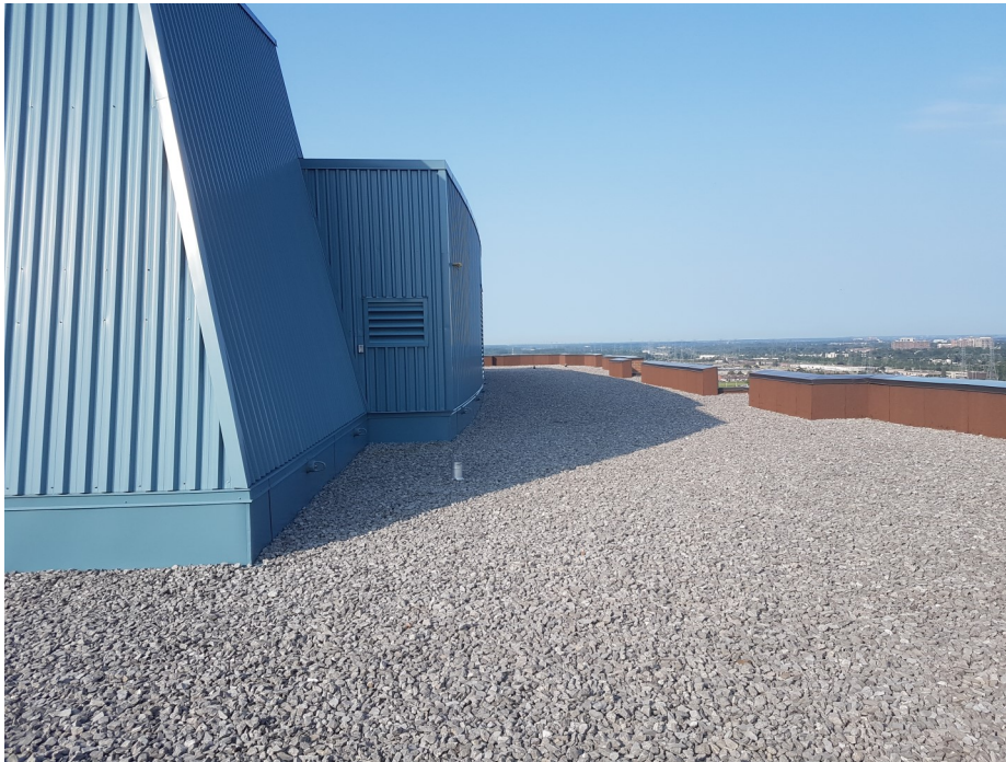
3. General view of inverted roofing system and the mechanical penthouse aluminium siding
