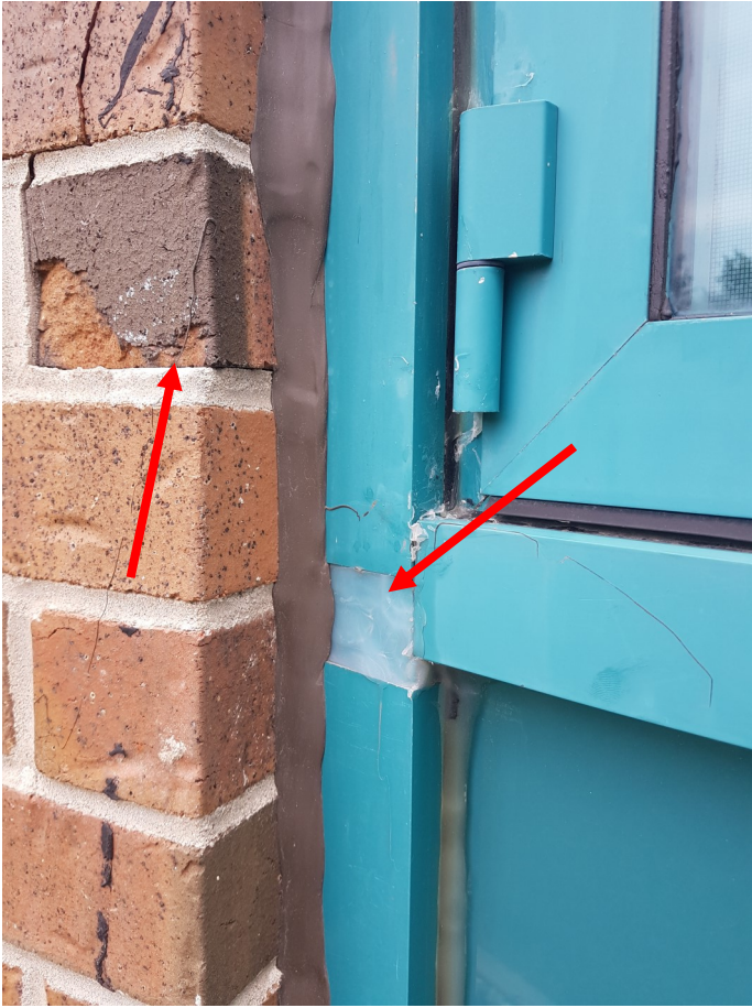
9. Showing punched widow frame silicone sealant repairs and localized masonry veneer delamination
