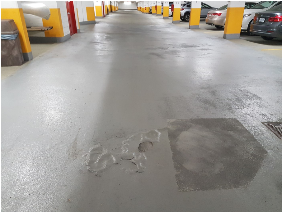
4. Showing traffic bearing membrane delamination and previous repairs within the parking garage
