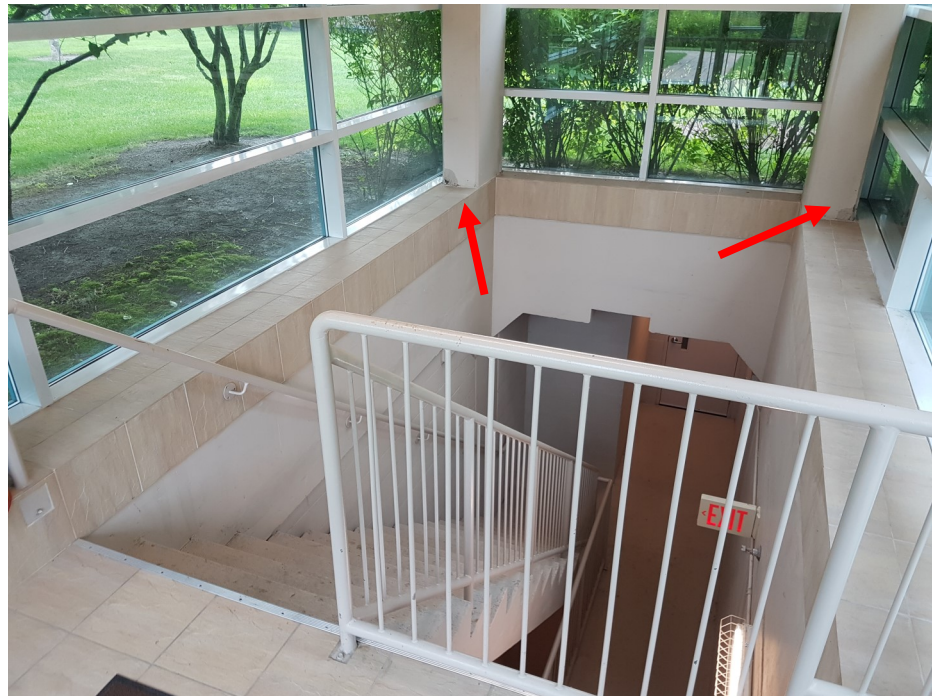
10. Showing condition of podium stairs with localized concrete column delamination
